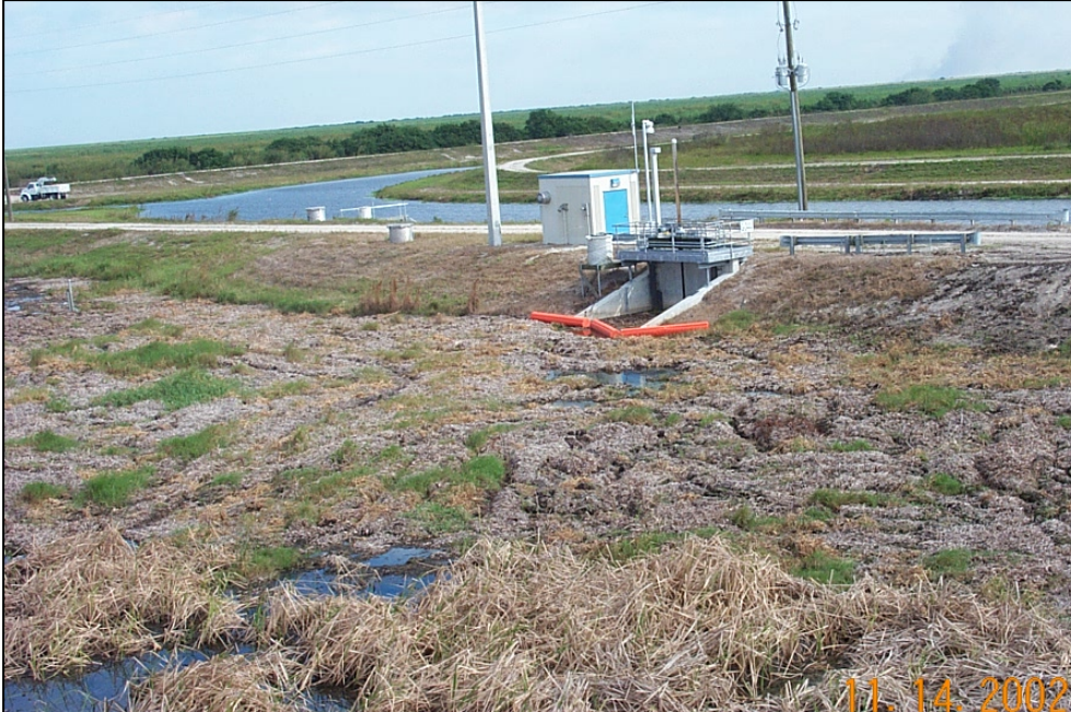
Figure 7-4. Example of FAV blocking a water control structure in STA-5.
