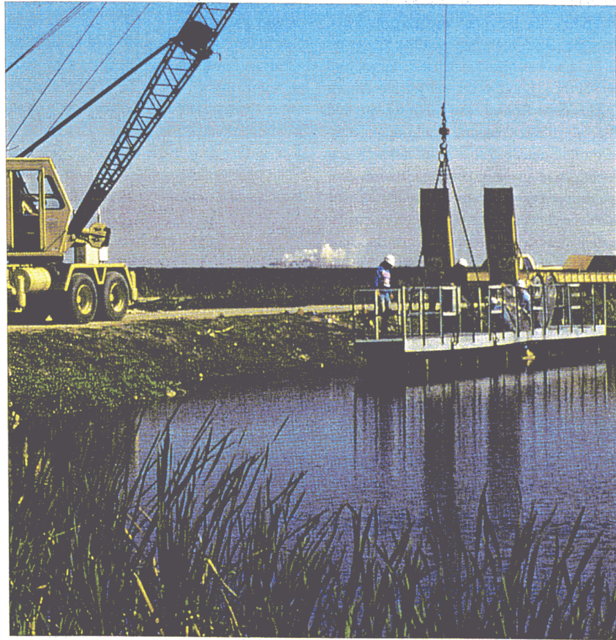
THIRTY-EIGHT 72 IN. CULVERTS WITH FLASHBOARD RISERS LOCATED ALONG THE INTERIOR LEVEES PROVIDE INTERNAL WATER CONTROL WITHIN THE EVERGLADES NUTRIENT REMOVAL PROJECT.
